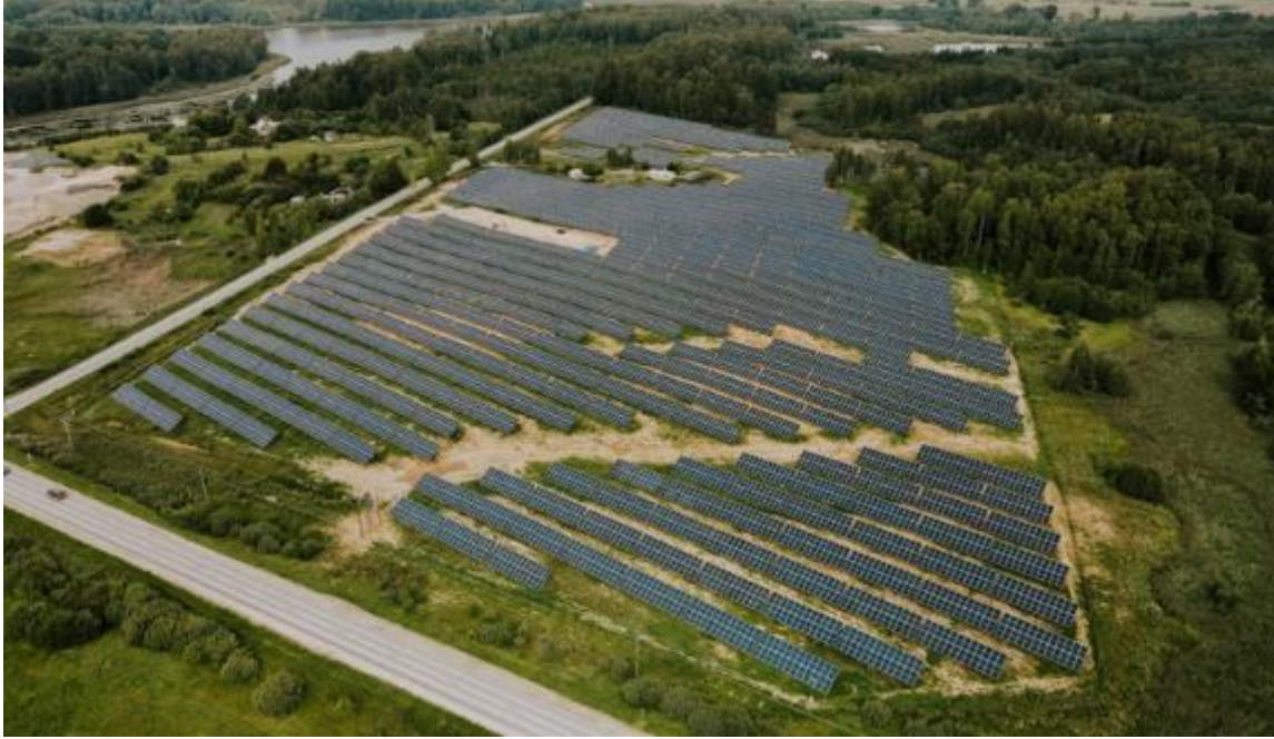
External park, 5 MW line (6.34 MW total)
